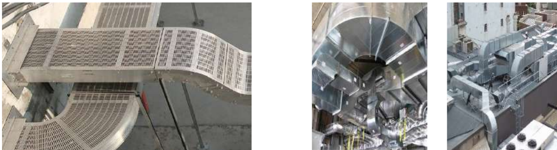
AC DUSTING SYSTEM
